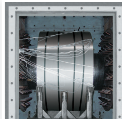
High Convection Vortex Flow system installed in the furnace
