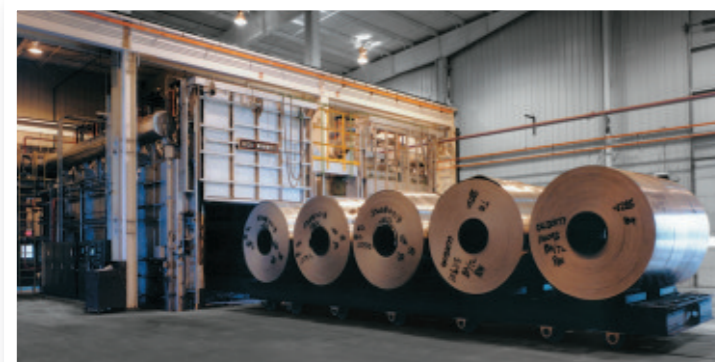
SECO/WARWICK's coil annealing multi zone furnaces
