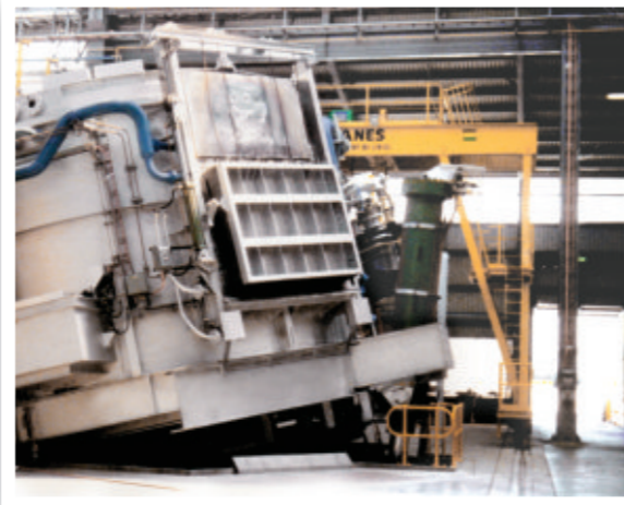
Round melting furnace in the tilting position
